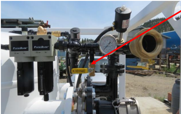
Control 1/4" Purge Valve
