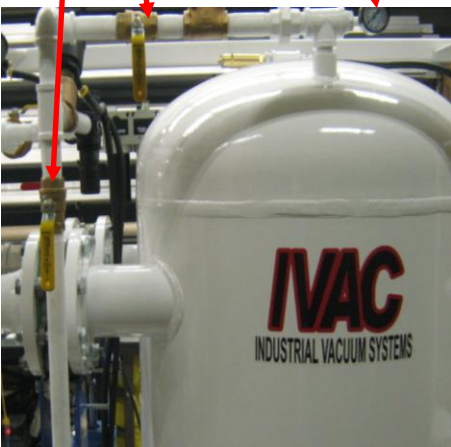
2-1" ball valves Tank pressure gauge
